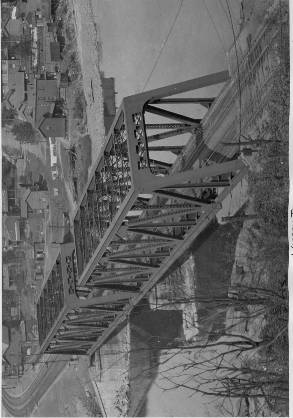
WARREN TRUSS Br. No. 92 Cumberland Div. - Crossing Cheat River at Rowlesburg W. Va.
