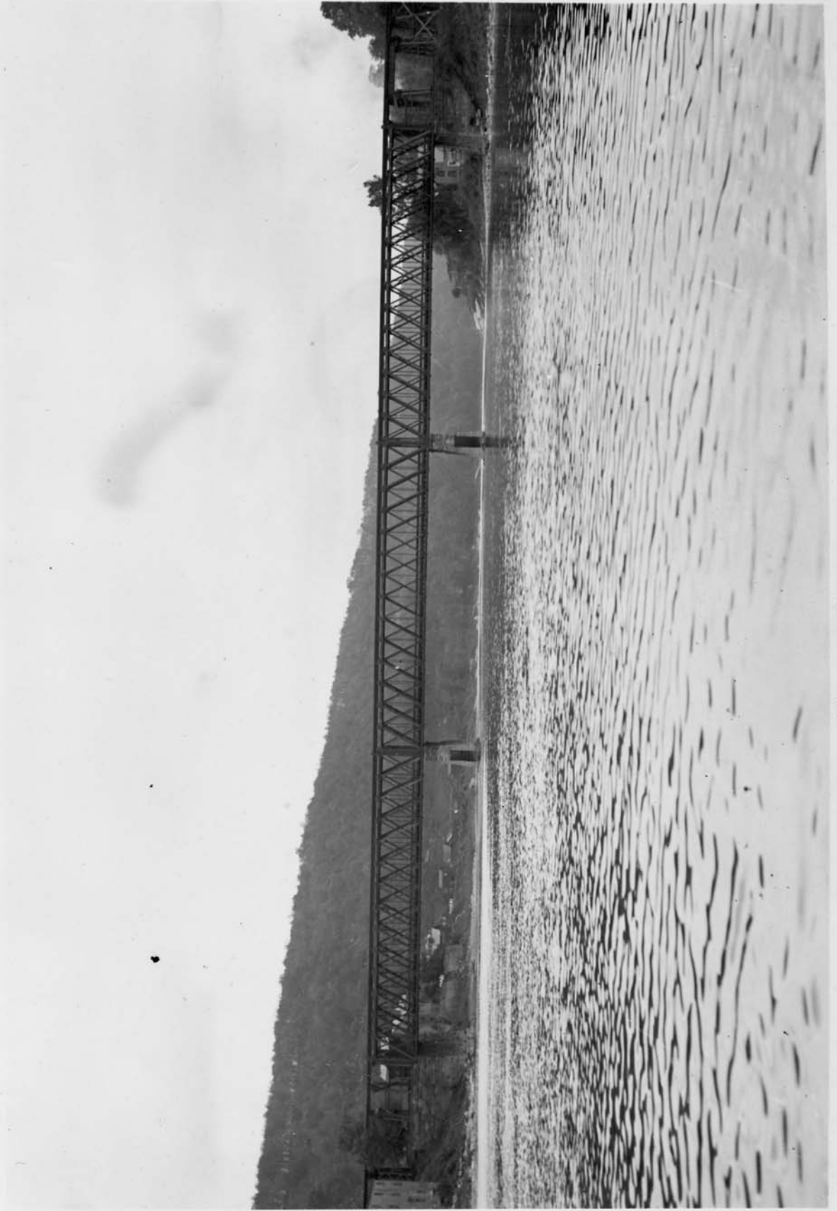
HOWE TRUSS Br. No 467 Pittsburga Div. crossing Allegheny River at Foxburg, Pa.
